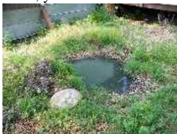
Septic flowing on surface.
